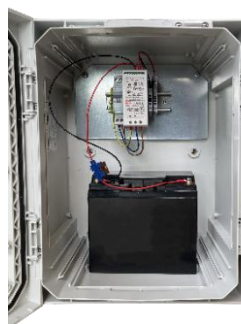
Street Lighting box
