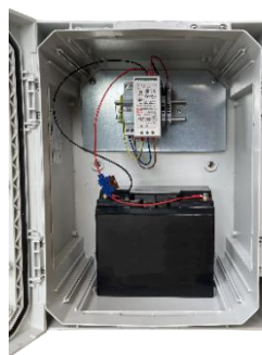
Street Lighting box
