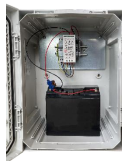
Street Lighting box
